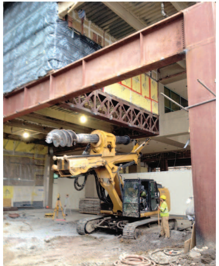
CZM EK125 Drill Rig with boom down and in route to next drilling location.
