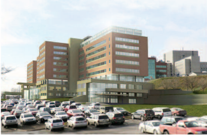
Thousands of automobiles adjacent to the job site made for careful planning when materials and equipment entered the work area.
