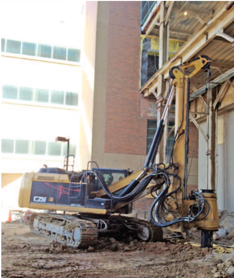
Brayman operator drills at a depth of 25 ft using a CZM EK125 Drill Rig with 42 inch diameter shaft.
